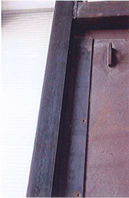
Posttest Photograph of Door Edge Plate Connection Failure
